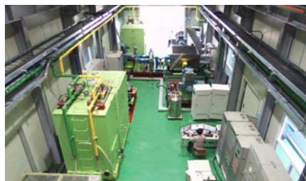
Fig. 2. (Combined environment)Hybrid dynamometer test equipment
